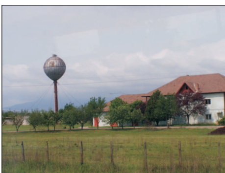
Phot. 24. Tower reservoir in a poor technical condition (photo: J. Pawełek)
