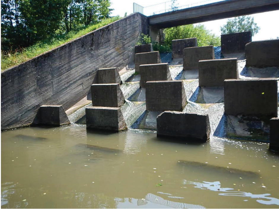
Figure 2. An example of interlocked-carpet block ramp (BR) of a Peterka kind constructed on Lubenia stream, phot. A.Radecki-Pawlik
