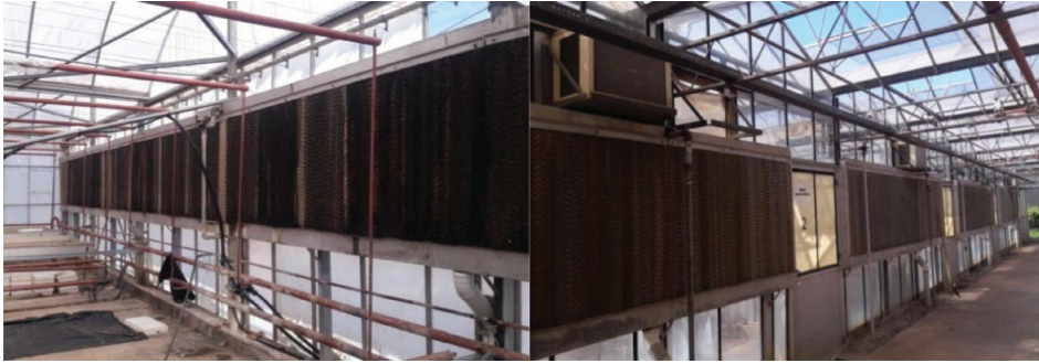
Figure 9. A view of fan-pad system in greenhouses in the study area
