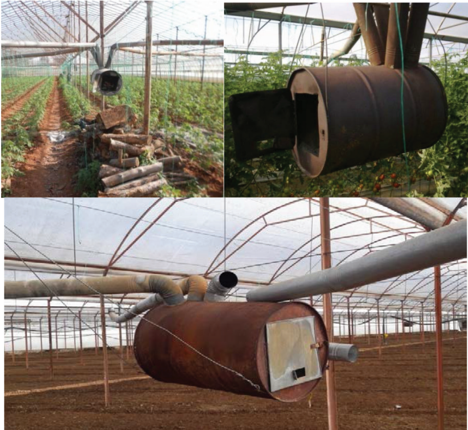
Figure 4. A view of stove used in greenhouse heating
